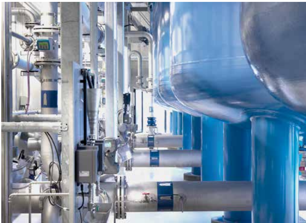
INTERIOR AT THE MARBJERG WATERWORKS – PHOTO BY MARTIN DYRLØV
