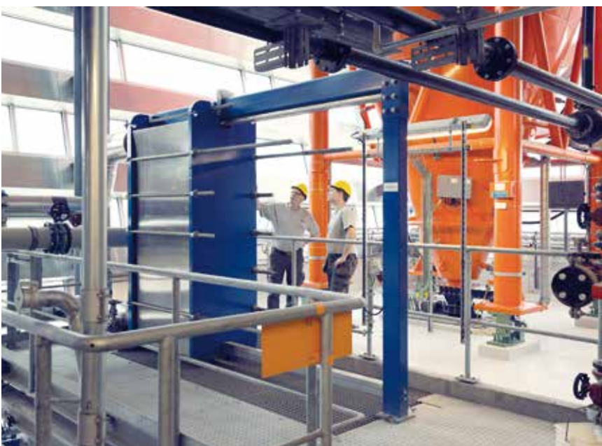
DISTRICT HEATING AT BIOFOS WASTEWATER TREATMENT PLANT “LYNETTEN” – PHOTO BY HVIIDPHOTOGRAPHY
